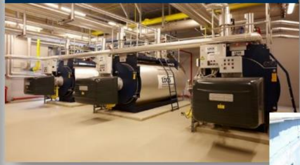
Gas boilers 3 x 2,5 MW
