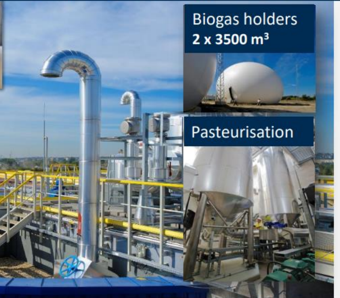
Thermophilic anaerobic digestion 3 x 6000 m 3
